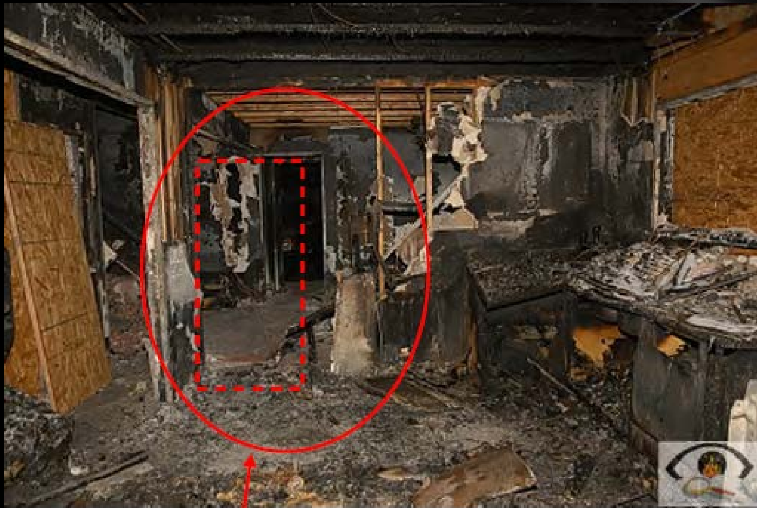
Image 2: The area of origin was at the west wall of the main floor kitchen where the refrigerator was located.
